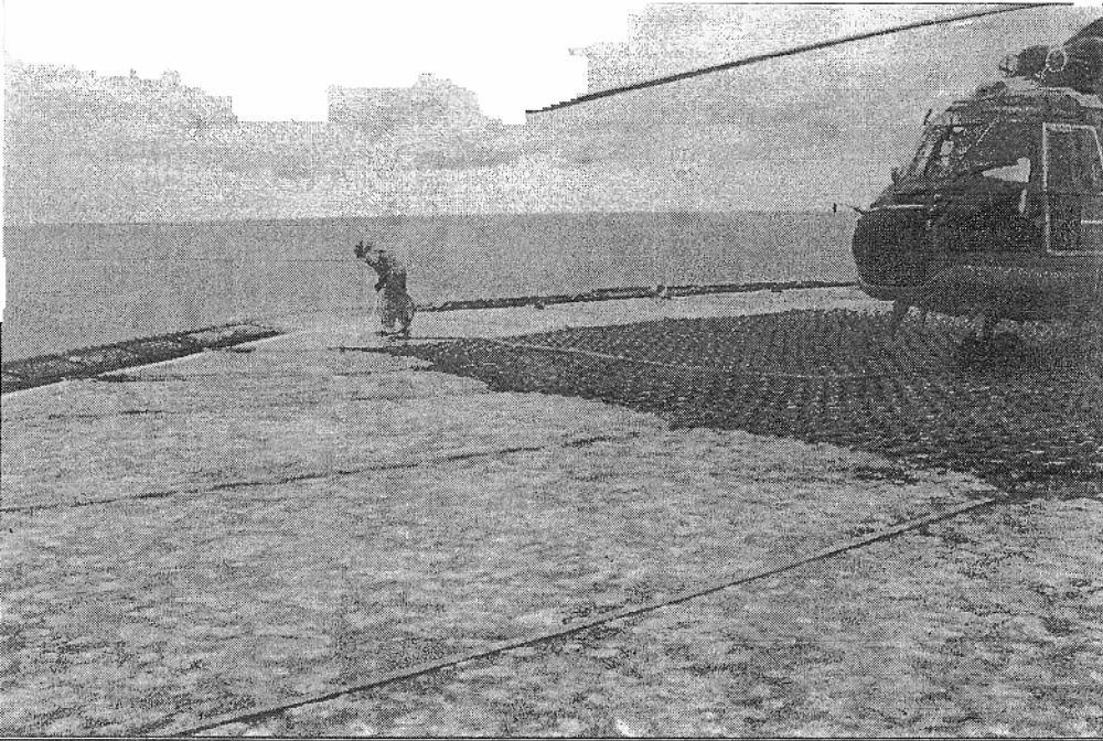
Figure 10.2 An Example of the effects of Guano Infestations on a Helideck Surface (Photograph courtesy of TotalFinaElf)
